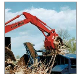
Wood Waste Handling
